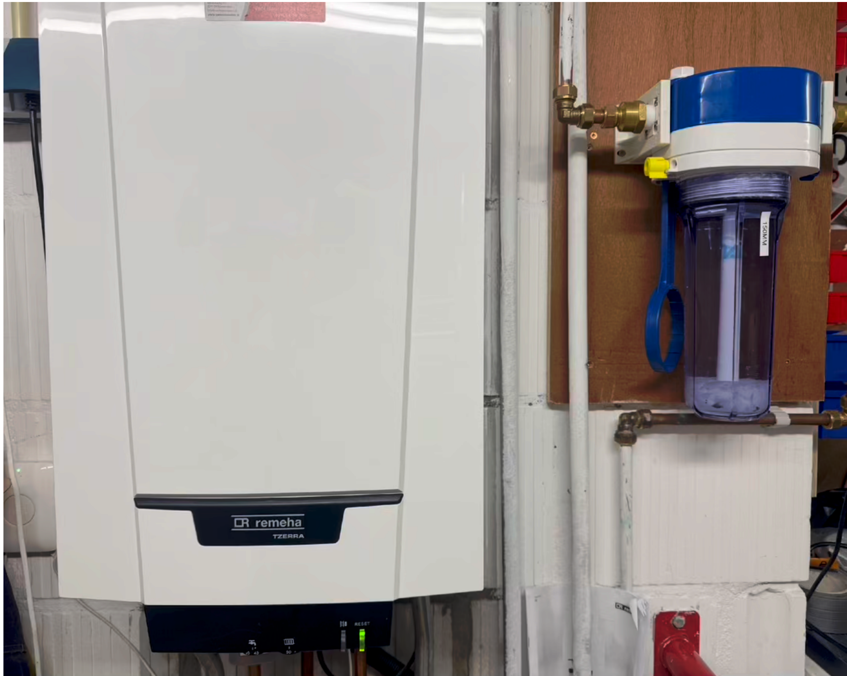
Gas heating system set to 45 degrees with Sensiblue, saving 12-18% gas use on showering.
