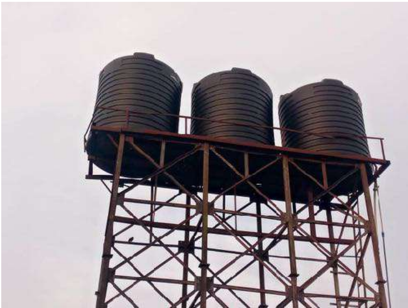
Water storage tanks, filled with borehole water. System is gravity fed.
