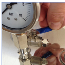
Purge air robinet 4-6 mm
